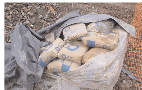
Damaged paper packaging on building site.
