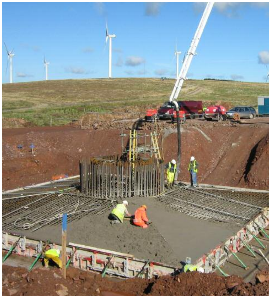
The base for a new wind turbine under construction at Whitelee wind farm
